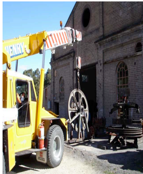
Sections of the winder being unloaded in May 2006.
